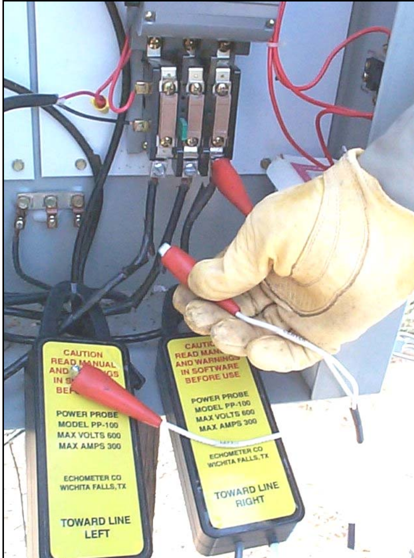
The above picture shows the Model 100 power probes correctly installed in the switch box.
