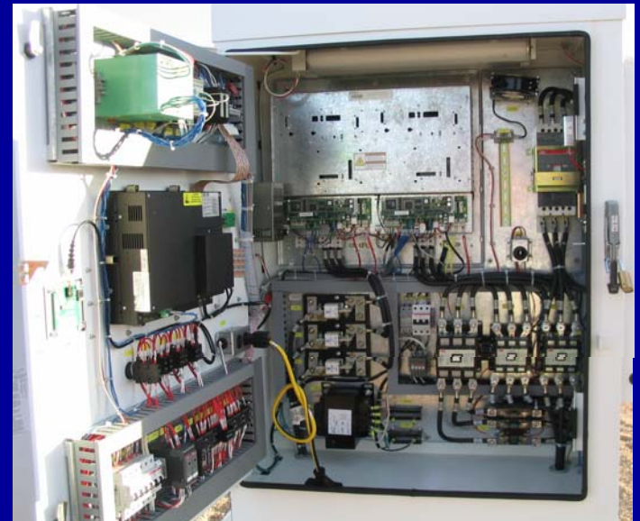
Used ABB VSD to Change SPM No Sheave Change ~ few Seconds
