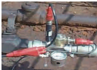
Well Analyzer Gas Gun & PT
